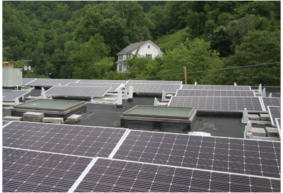
Solar panels have been installed at Homes Inc. in Whitesburg, KY. Similar panels will soon be installed at the Middlesboro community center © Mountain Association
