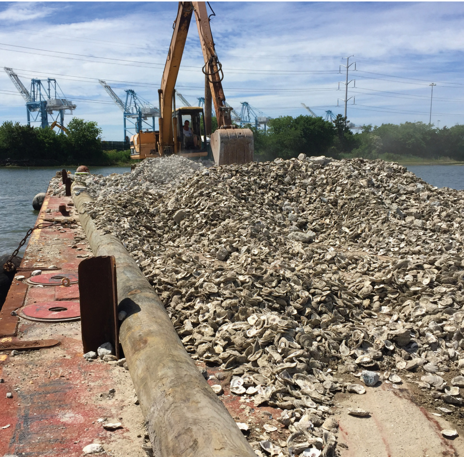
Figure 5.6: Barge deploying shell and stone to restore shellfish reefs as part of the Elizabeth River Project, Chesapeake Bay, USA. Photo: Joe Rieger.
